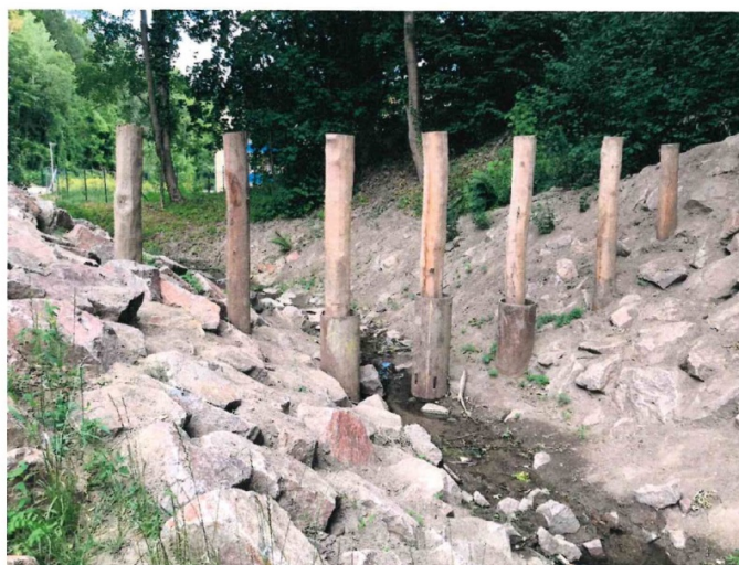
Vertical wooden racks acting as a debris barrier Source: M. Sura, Hoch- und Tiefbau GmbH
